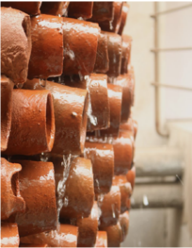
fig. 27 (Deki Cooling Installations, n.d.)
